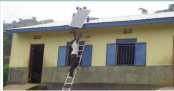
Photograph: Solar panels at Musasa Primary School
